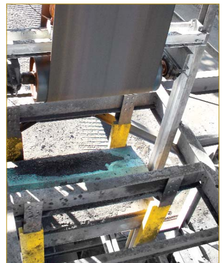
Close-up of the Technogrid® installation from the top. Note the guide channel on the right hand side for the counter weight.
